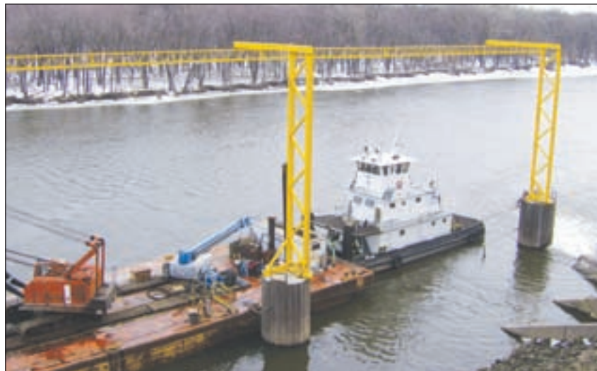
Overhead truss fall protection system installed at a marine terminal. (Photo courtesy of Diversified Fall Protection)
