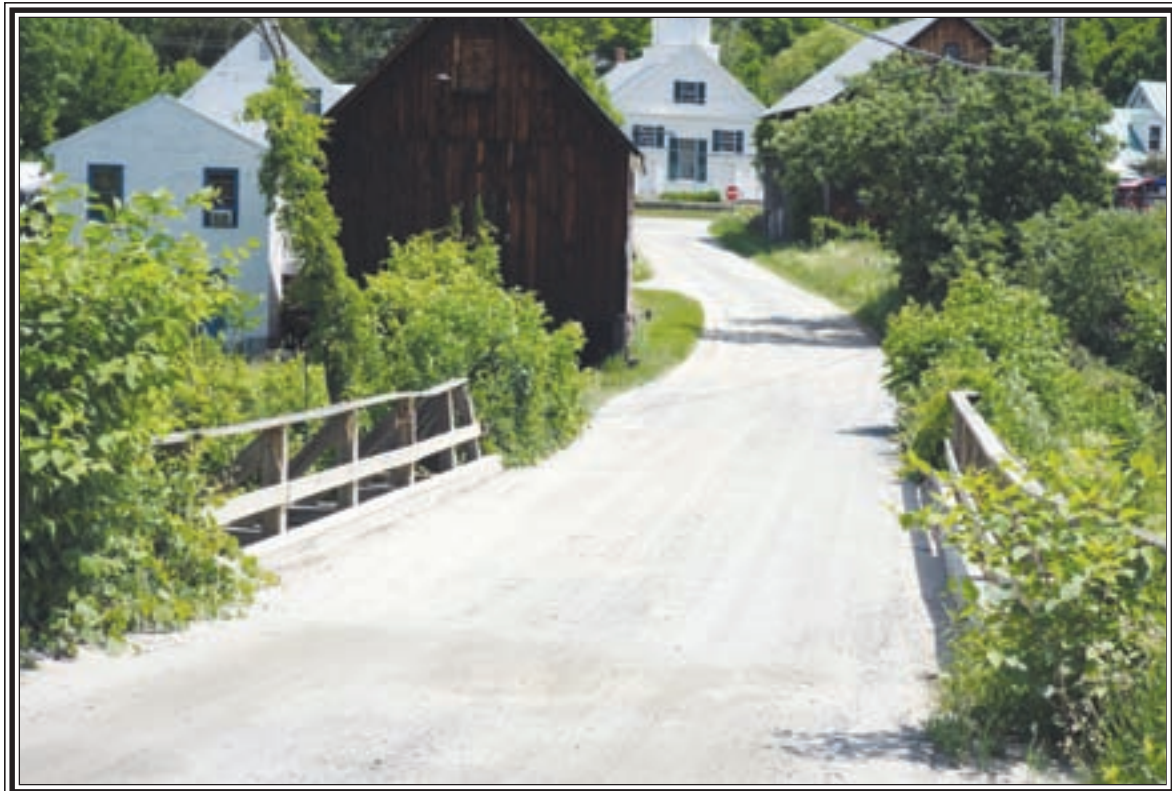
This familiar scene in Waits River could look different later this year as the bridge in the foreground undergoes repair work with metal guardrails set to replace the deteriorating wooden ones.
