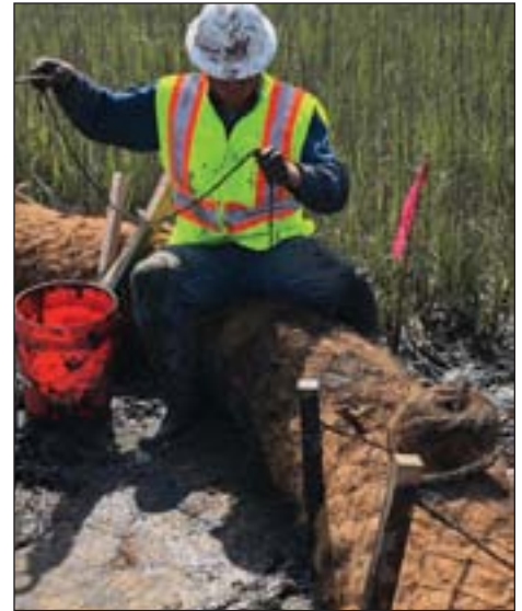
Coconut coir logs are placed around the wetland disposal area to keep the material from running off into adjacent waterways and marsh. The coconut coir logs for this project required the use of a biodegradable netting instead of plastic to ensure the coirs completely degraded.
