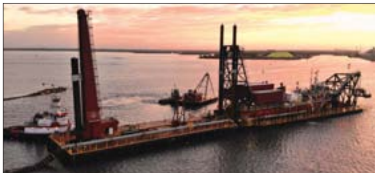
TOP: GLDD was able to maneuver the cutter head on the dredge Carolina into the berthing areas in Tampa Harbor getting within five inches of the bulkhead without damaging the structure.
