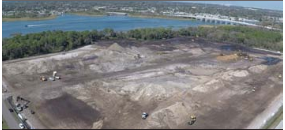
In late 2018, Gator Dredging started work at Lake Seminole in Florida. Construction of a dredged material placement site will be completed in August 2019, after which dredging will begin.
