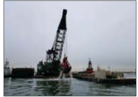
On April 1, the Dale Pyatt, a large class bucket dredge of contractor Cashman Dredging works in Boston Harbor in Massachusetts. The dredging work is a joint venture between two companies, the Dutra Group and Cashman Dredging.
