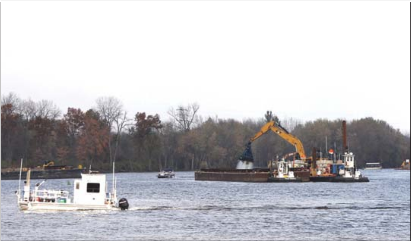
GE performed dredging at the Hudson River PCBs Superfund Site between 2009 and 2015. It dredged a total of 2.75 million cubic yards of contaminated sediment from the 40-mile stretch of the Upper Hudson River.
