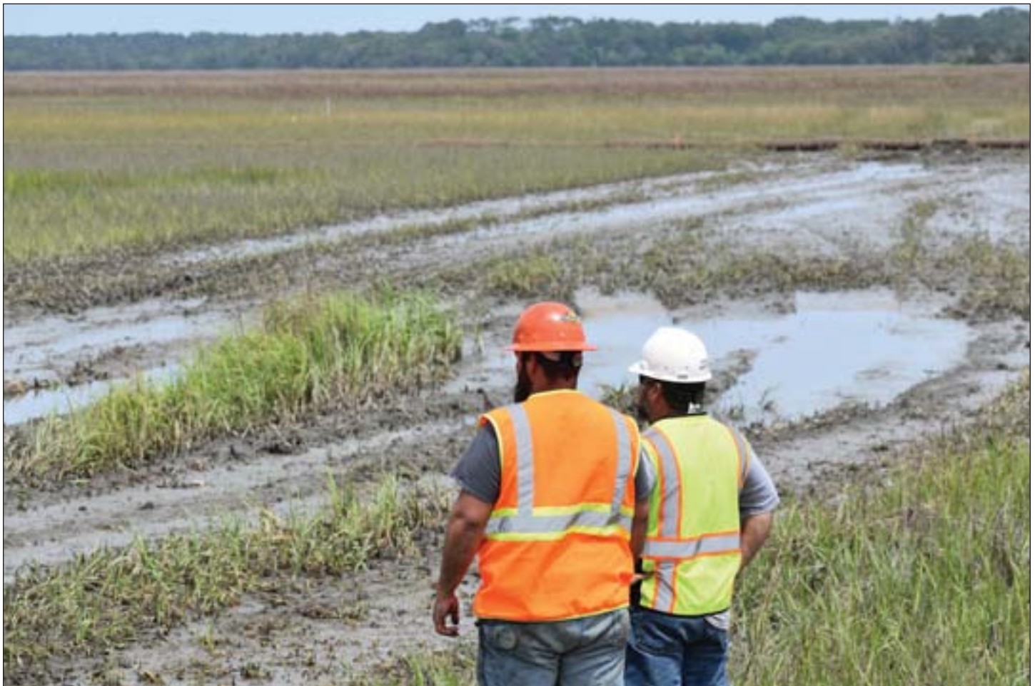
Material dredged from Jekyll Creek is being rainbowed onto this wetland area to raise the elevation of the land while maintaining marsh grass growth.
