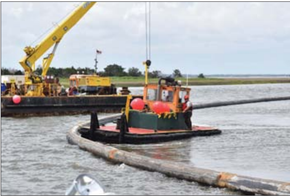
Dredging of Jekyll Creek is part of a pilot program where material will be sent via pipe to both a deep hole in the channel and onto nearby wetlands.
