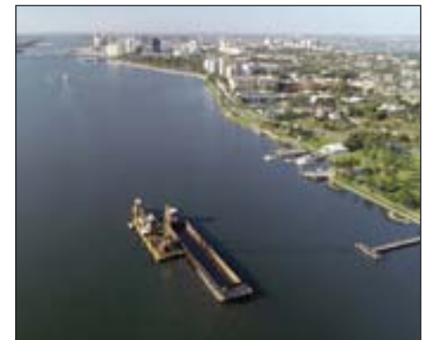
Orion Marine Construction is dredging a portion of the Intracoastal Waterway channel to its federally authorized depth.
