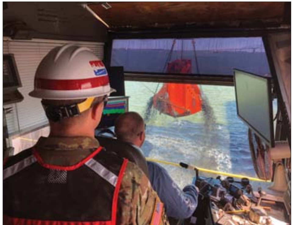
U.S. Army Corps of Engineers Baltimore District Deputy Commander Lt. Col. Geoffrey Kuhlman looks on aboard a Norfolk Dredging Company dredge, as a load of material is pulled from the bottom of Curtis Bay Channel in Baltimore Harbor on March 19. The Corps contracted with the company for maintenance dredging of the channels associated with the Baltimore Harbor. Curtis Bay Channel was one of six dredged, during which crews removed nearly 2.6 million cubic yards of material from channels. (Photo Credit: Chris Gardner, U.S. Army Corps of Engineer Baltimore District)
