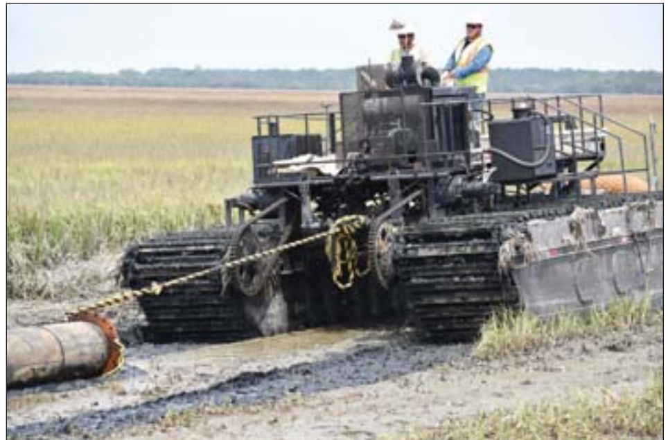
Cottrell Contracting had to minimize the use of heavy equipment as they laid pipe in the wetland disposal area.
