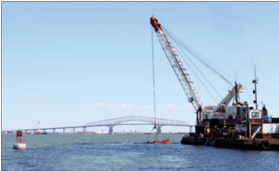
A U.S. Army Corps of Engineers contracted dredge operated by Norfolk Dredging lifts material out of Curtis Bay Channel in Baltimore Harbor Tuesday March 19, 2019 as part of maintenance dredging of channels associated with the Baltimore Harbor and Channels Project. Curtis Bay Channel was one of six dredged during the Fiscal Year 2019 maintenance cycle, during which crews removed nearly 2.6 million cubic yards of material from channels to ensure continued safe navigation for vessels traveling to and from Port of Baltimore facilities. (U.S. Army photos by Becca Nappi)
