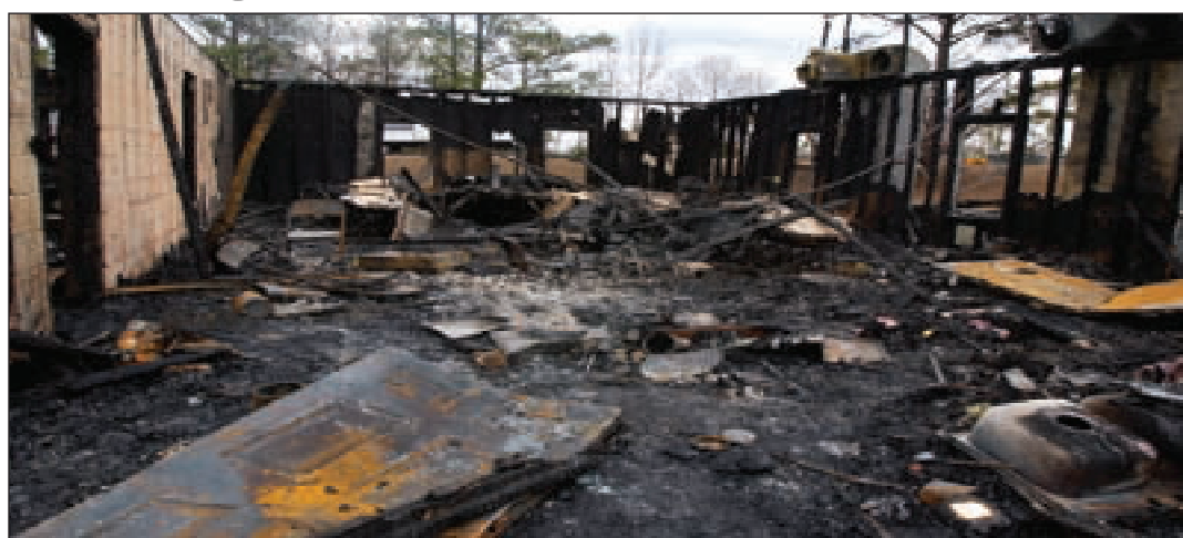
Damage caused by a fire at Beaverton Freewill Baptist Church is shown Feb. 12, in Beaverton. Investigators have determined that the fire was arson.
