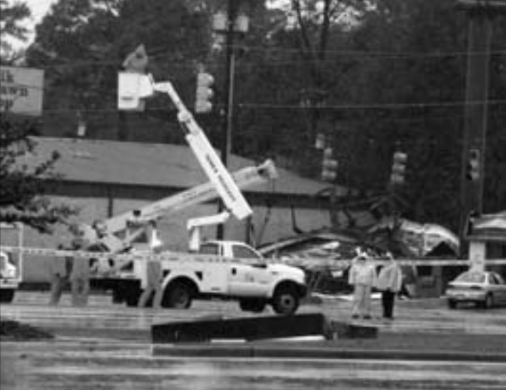
Alabama Power workers act quickly to repair damaged power lines at the intersection of 15th Street East and McFarland Boulevard on Tuesday afternoon.
