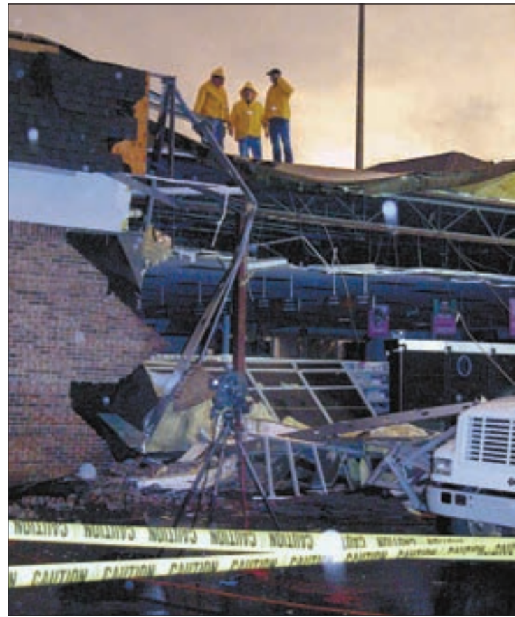
Check out The CW photo gallery of the tornado damage online at www.cw.ua.edu .
